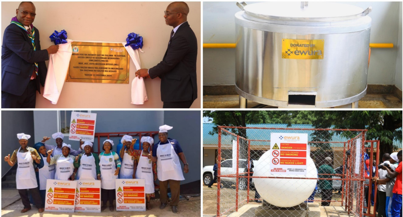
Figure 36: EWURA Donating the Domestic LPG Bulk Storage and Kitchen Installation to Morogoro Secondary School
